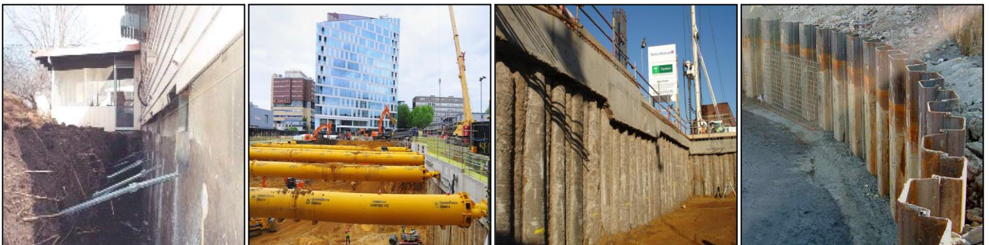
Fig. 6.2: (a) Anchored wall, (b) Braced excavation, (c) Bored pile, (d) Sheet pile
