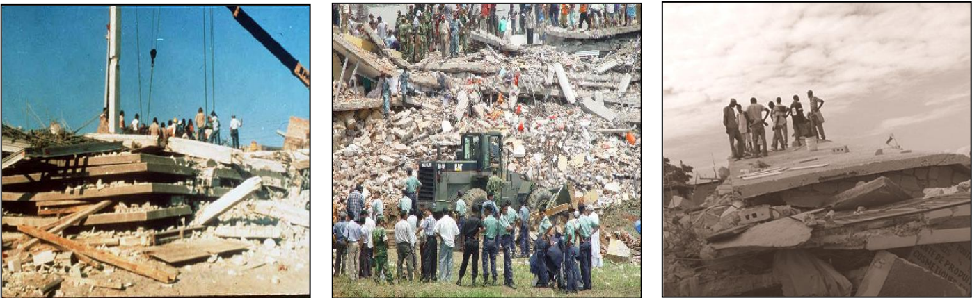
Fig. 2.11: Pancake failure of slabs in (a) USA (1981), (b) Bangladesh (2005), (c) Haiti earthquake (2010)
