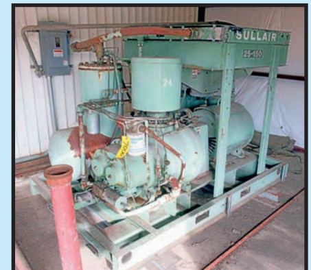
SULLAIR 25 HP ROTARY SCREW AIR COMPRESSOR
