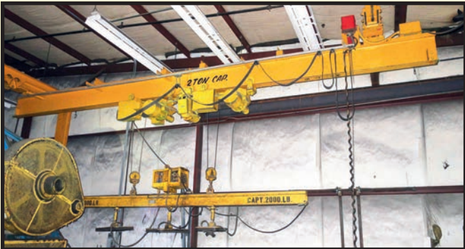
CUSTOM 2 T. X APPROX. 24' SPAN OVERHEAD BRIDGE CRANE SYSTEM
