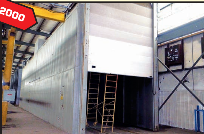
JBI 14'W. X 18'H. GAS FIRED PAINT BAKE OVEN
