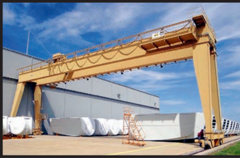
P&H 88 T. CAP. X 77' SPAN DOUBLE LEG GANTRY CRANE
