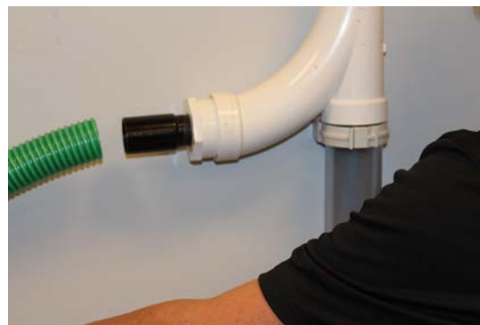
Figure 4.7-8: Flexible Intake Tubing
