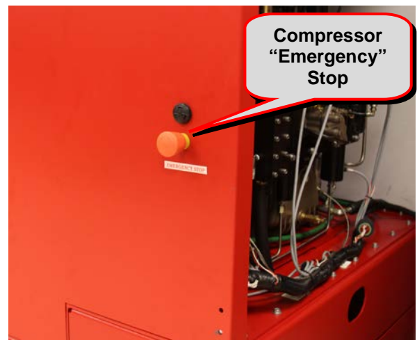
Figure 3.4-2: Compressor Emergency Stop
