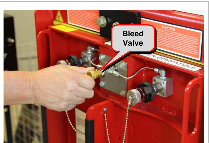
Figure 3.6-1: Open Bleed Valve
