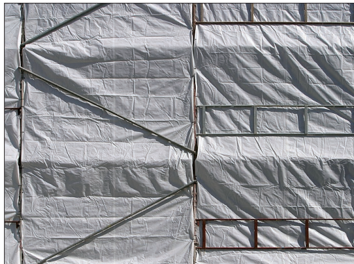
Exercise caution with wrapped scaffolding due to wind conditions.
