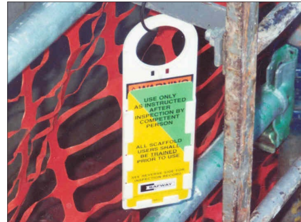
Tags stating the current status of the scaffold is a best practice among many companies.
