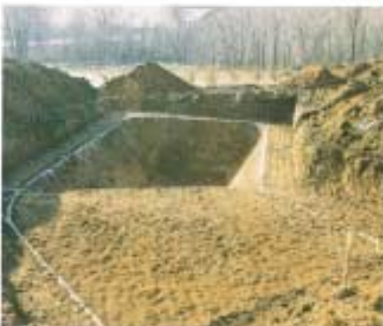
The pool is excavated to the dimensions provided on the Fox drawing.
