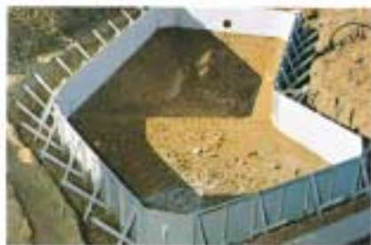
Fox Panels and Braces are assembled and the pool walls are plumbed and leveled. Several tons of concrete are poured around the Braces and Panels, to serve as a permanent footer. Note the bulwark of braces.
