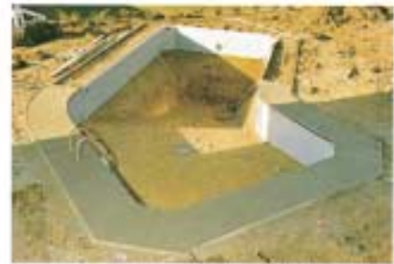
Here the walls have been backfilled and the decking partially poured, visual proof that the pool can be backfilled and the deck poured with no need to equalize backfill with internal water pressure.
