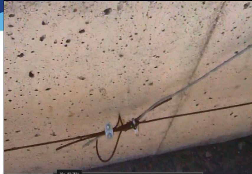
Rusted cable repaired by attaching new cable to old rusted piece
