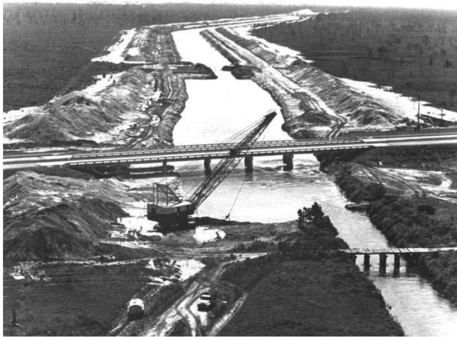
Figure 6-7. Construction of the U.S. 19 bridge over the Cross Florida Barge Canal in Inglis, Florida (late 1960s). Courtesy of the Florida State Archives.
