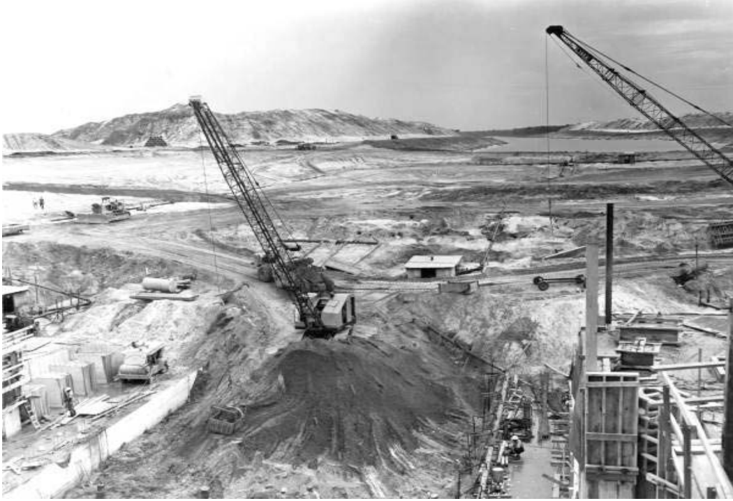
Figure 6-8. Construction of the St. Johns Lock, late 1960s. Florida's terrain has been transformed beyond recognition. Courtesy of the Florida State Archives.
