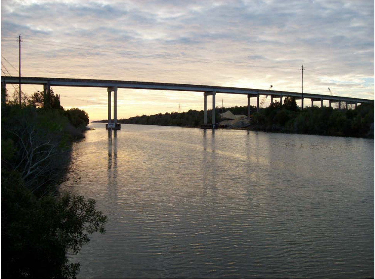
Figure 7-3. A view of the U.S. 19 bridge over the Cross Florida Barge Canal at Inglis, near the Gulf of Mexico. Photo by Peggy Macdonald.
