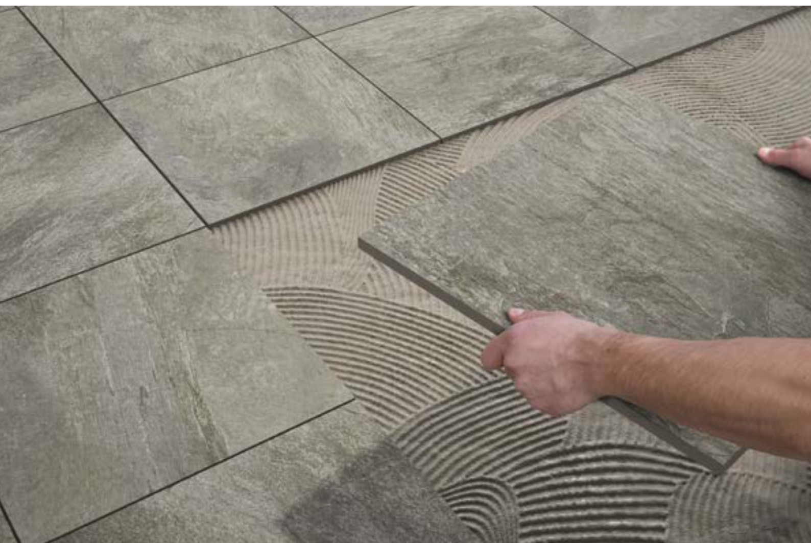
Floor tiles: MY EARTH OUTDOOR grey multicolour on cement screed
