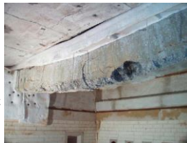
Failure of an RC beam after fire test inside the furnace, showing flexural cracks
