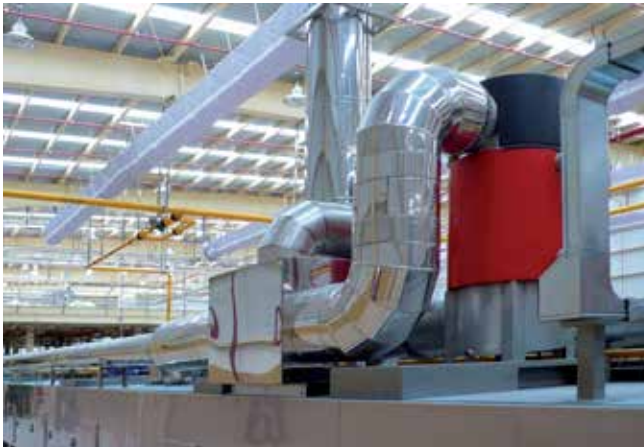
Heat recovery system channels heat from the oven back into the plant
