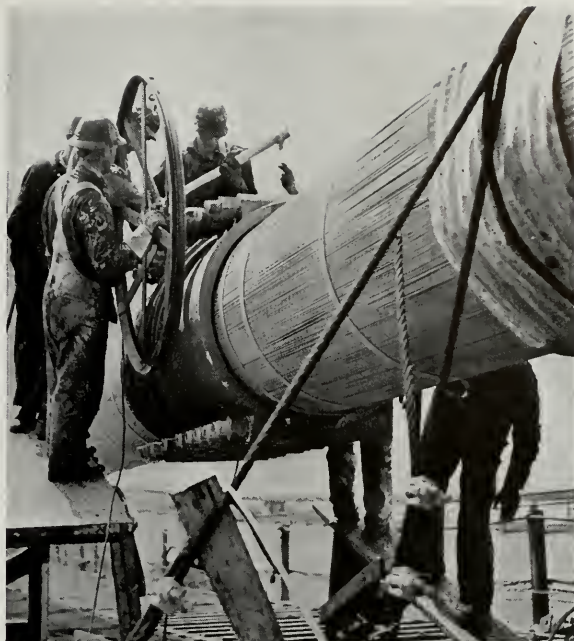
The giant 36-inch cables of the Golden Gate Bridge were "squeezed" together by powerful machines. Photo shows workmen removing spinning apparatus preparatory to binding with final wrapping.
