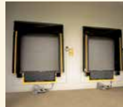
Rolling Service Doors
