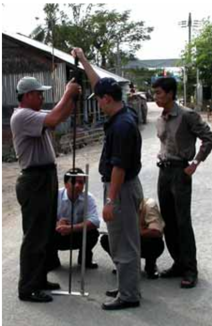
Figure 9.7: Dynamic cone penetrometer in use for measuring the strength of an existing pavement
