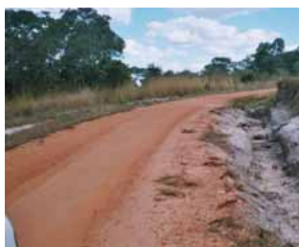
Figure 11.3: This side drain is eroding severely. Access along the road may soon be lost. Scour checks should be constructed
