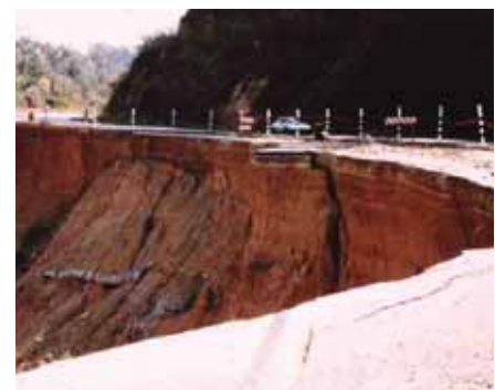
Figure 5.3: Some areas are prone to landslides
