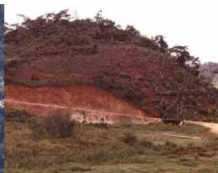
Figure 5.4: Major cuttings are sometimes unavoidable on trunk roads and on rural access roads
