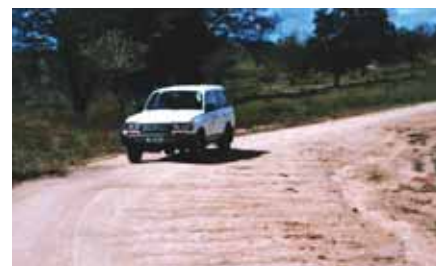
Figure 11.1: Transverse erosion on a super-elevated curve
