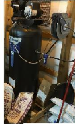
Air Compressor for SandBlaster
