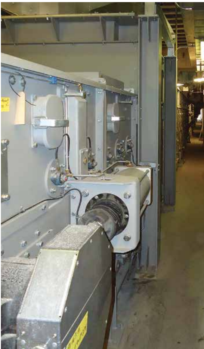
PICTURE 4: ECOBELT® WA INSTALLED AT KEZO HINWIL #1.
