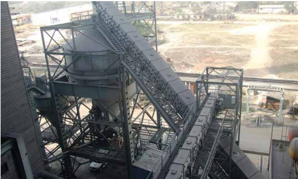
FIGURE 4: THE MAC® SYSTEM IN DURGAPUR P.P.
