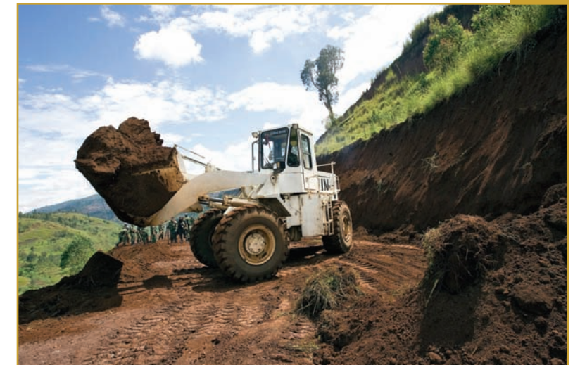
Military personnel of the Chinese engineering company of the United Nations Organization Mission in the Democratic Republic of the Congo (MONUC) operate a tractor to rehabilitate a 1.8 kilometer long road to allow greater access to the Ruzizi One Dam Power Plant, the only source of electricity for the east of the country. (UN Photo #185627 by Marie Frechon, April 2008)
