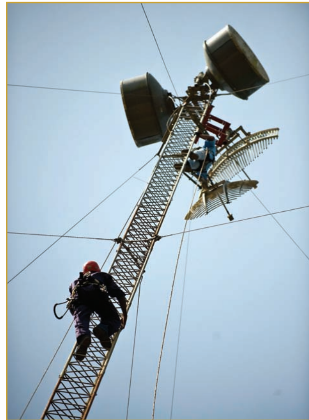
Electrical technicians of the Communications Information Technology Section of the United Nations Mission in Liberia works on the radio tower in the Bomi County. (UN Photo #325801 by Christopher Herwig, February 2009)
