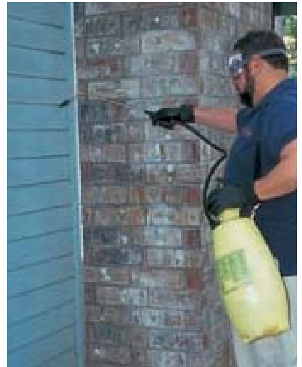
A garden sprayer is a cheap, portable way to apply stripper to shingle siding.
