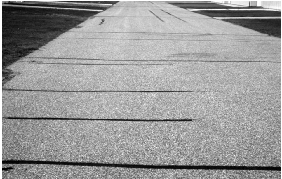
▲ Thermal cracks less than 10' apart. Slight raveling.
