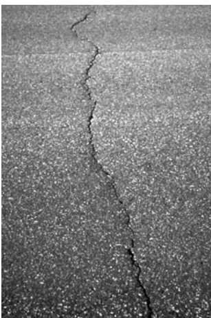
▲ Tight cracks less than 1/4" in width.
