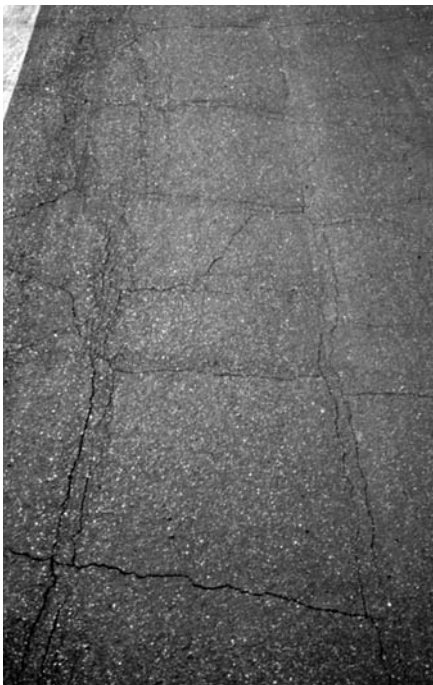
▲ Block cracking with cracks less than 5' apart.
