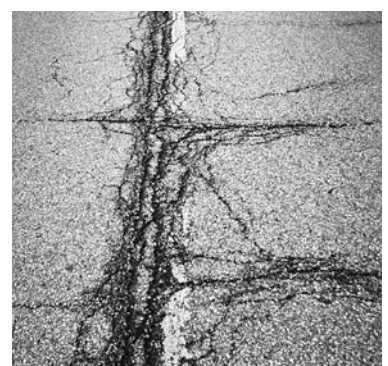
▲ Pavement ravels and erodes along open cracks causing deterioration.
