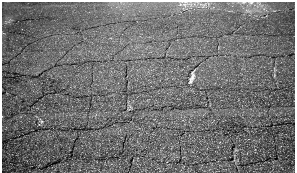
▶ Small blocks with open cracks.
