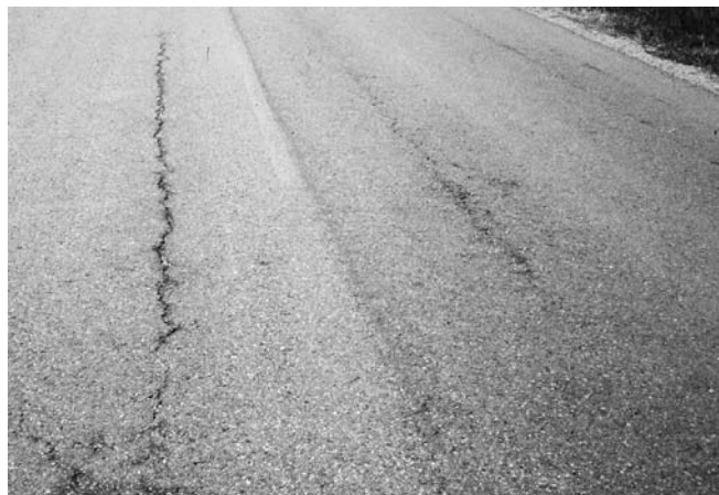
◀ Partially open 1/4" paving joint.
