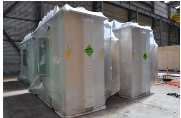
Figure 40: Nitrogen purged transformer furnished with gas cylinder
