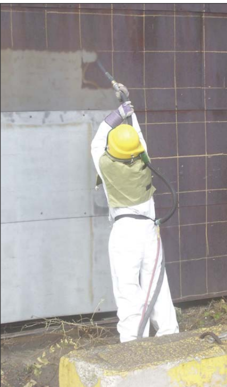
Productivity test, conducted under third-party guidance, on heavily pitted and rusted steel structure at a steel mill. Round and angular abrasives were tested for productivity and usage.
