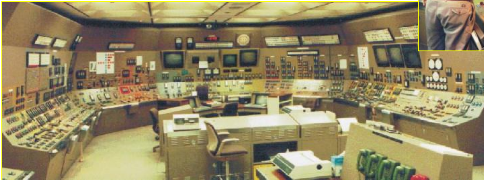
The Control Room (each Unit)
