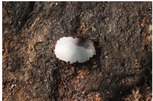
Figure 7: Photograph showing the hole in the tank bottom as viewed from the outside of the tank.
