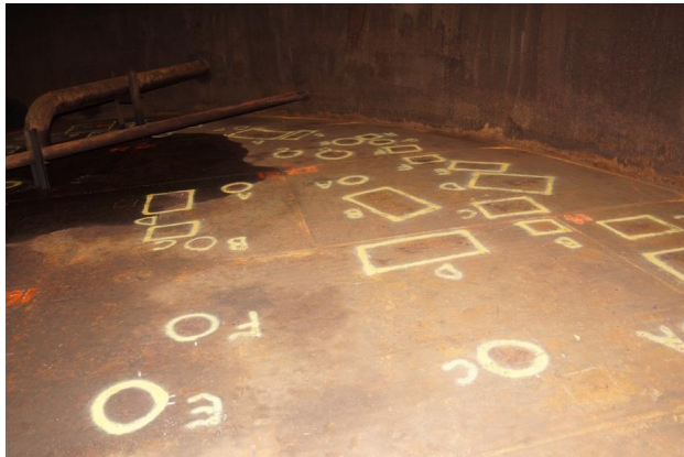
Figure 3: Photograph exhibiting perforated areas due to external corrosion. Perforated areas are randomly distributed.
