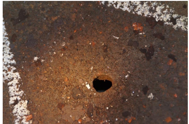
Figure 4: Close up of a perforated area
