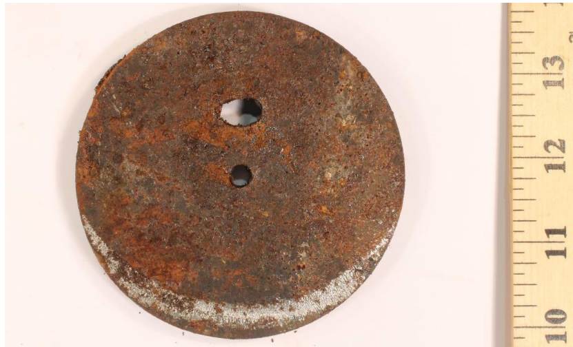
Figure 8: Photograph showing the hole in the tank bottom as viewed from the inside of the tank. Note-circular hole in center is a drilled hole.
