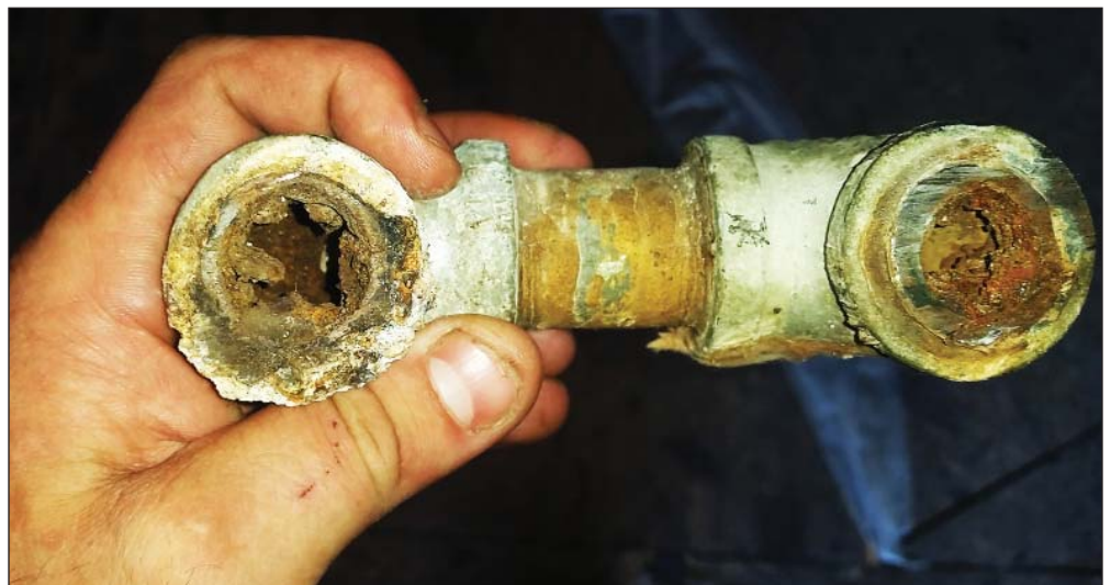
Typical condition of deteriorated pipe.
