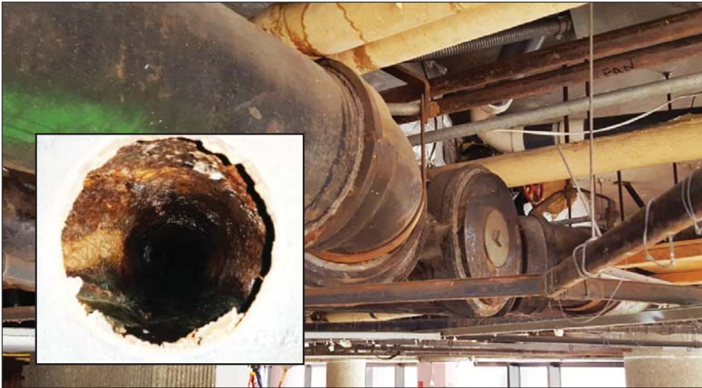
This is the main drain hub (Inset: the deteriorated and fragile conditions of these pipes can be seen from the inside).
