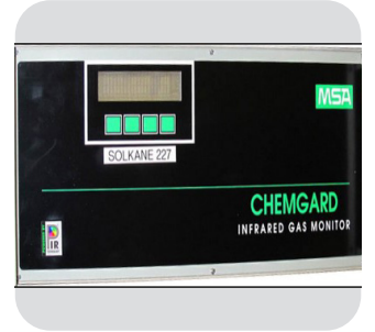
Gas Analyzers (H 2 , O 2 , CO 2 , CO)
