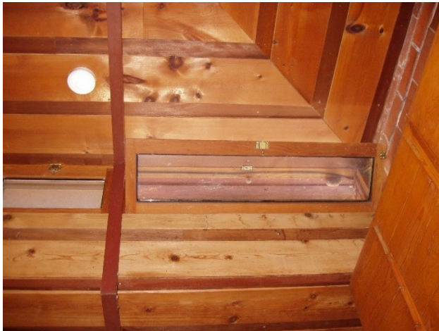
Figure 18 Clerestory window opening at Kitchen near the ceiling that creates a ventilating flue
