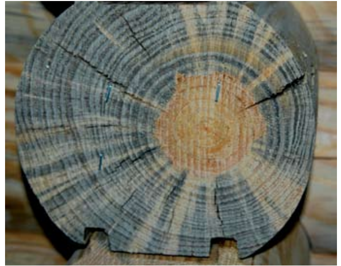
Bluestain has penetrated the sapwood of this pine log. The heartwood is not affected. The stain cannot be removed but the log is still structurally sound.
