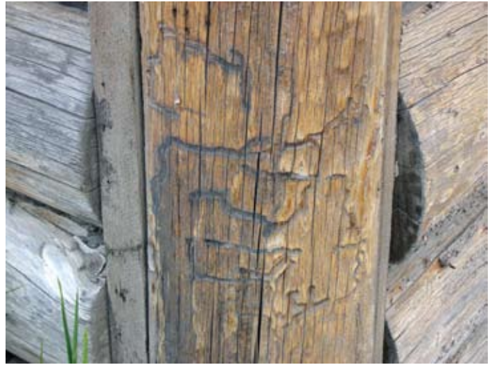
This log shows attack by bark beetles that occurred when the tree was standing. This log is still structurally sound and the beetles will not cause further damage.
