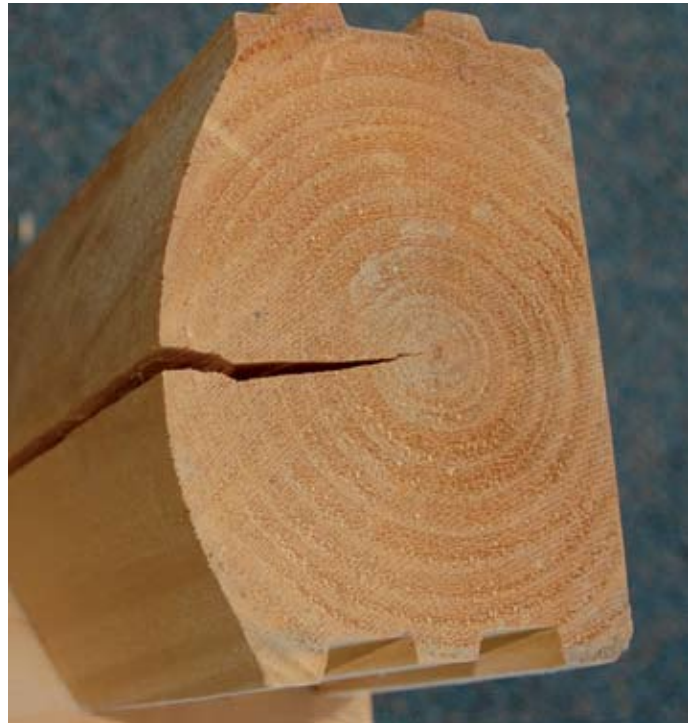
A check in a house log. This kind of split is the inevitable result of the normal drying process and the uneven nature of shrinkage in wood.
