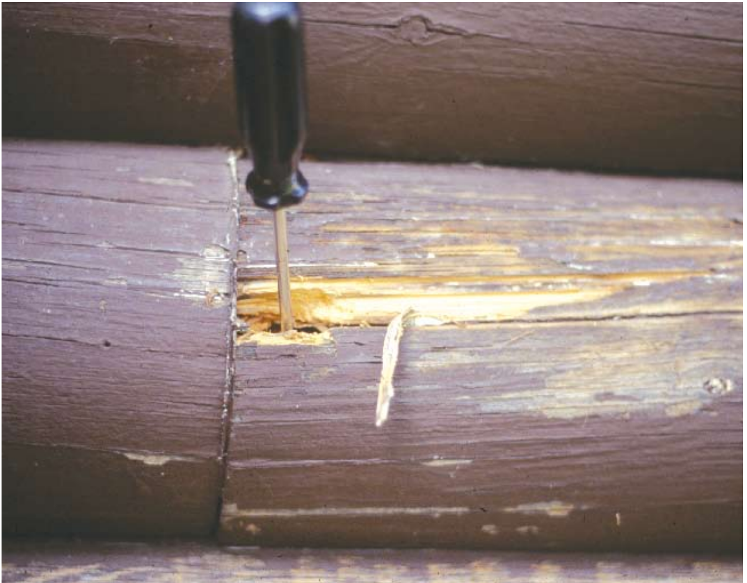
This log has been weakened by fungal decay. Butt joints are especially vulnerable areas because water that enters the joint is absorbed by the porous end-grain of the logs.
