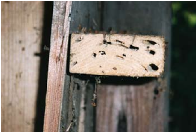
Drywood termite damage in a fence. Drywood termites inhabit the wood they are eating.
