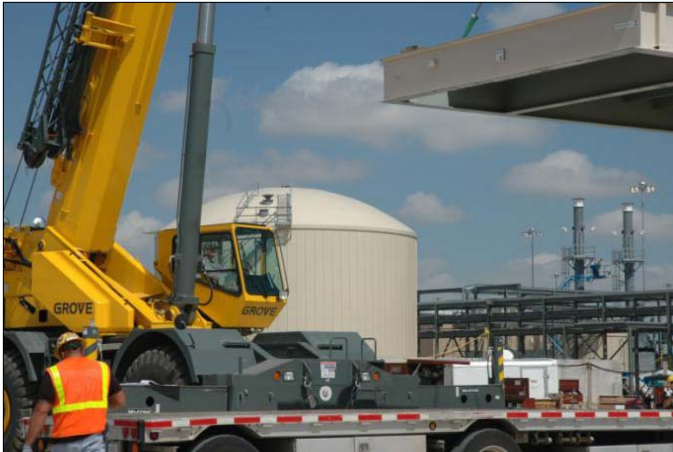
A base plate for the standby diesel generator is off-loaded in the utility area.
