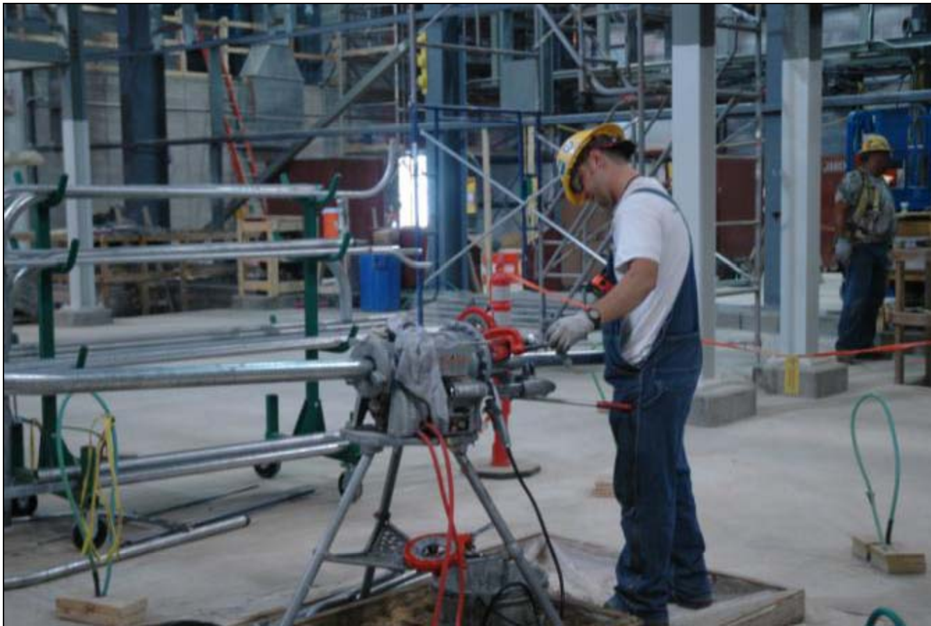
An electrician prepares conduit for electrical cable inside the Agent Processing Building.
