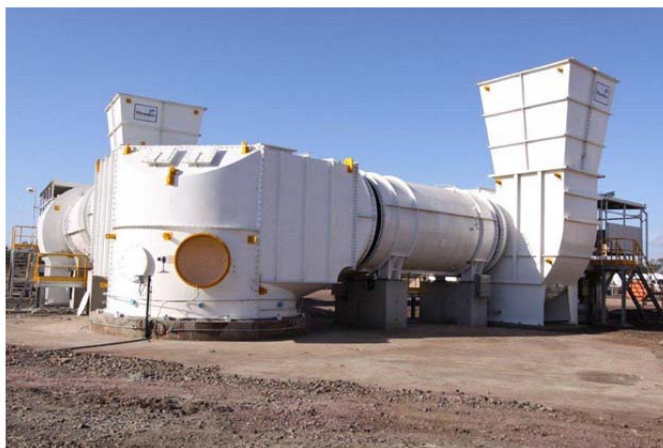
The dual mine fan at Peabody's North Goonyella Mine in Australia currently moves more than 290 cubic meters of air per second.
