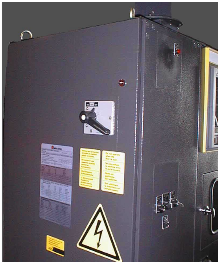
Pega 357 left side of electrical enclosure
