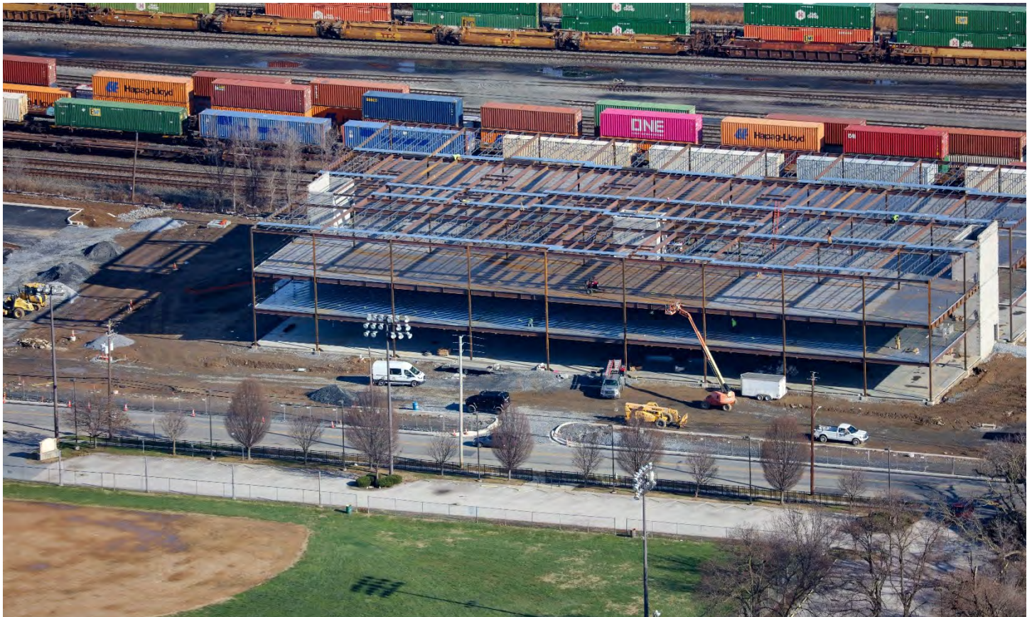
Future home of Department of Human Services and Office of Administration, 7th Street Harrisburg. Photo Courtesy of Hudson Companies.
