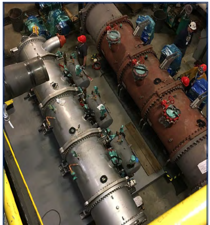
Installation of the central chiller plant as part of the Capitol Complex GESA project.
