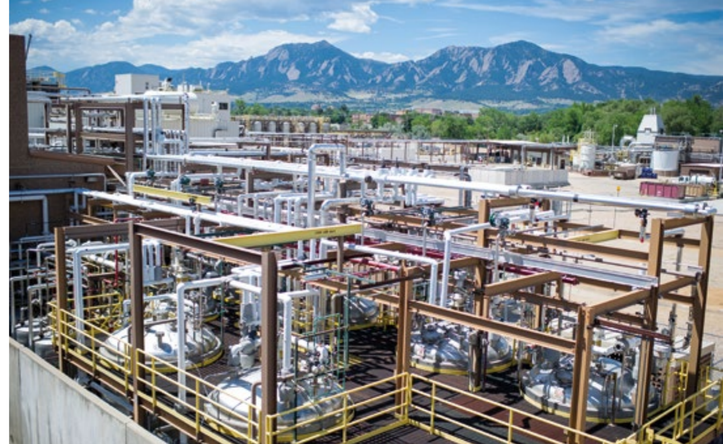
CordenPharma Colorado (USA) utilizes more than ten 50m 3 tanks to support our green manufacturing concept.
