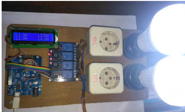
Gambar 4.20 Kondisi Lampu 1-4 ON
