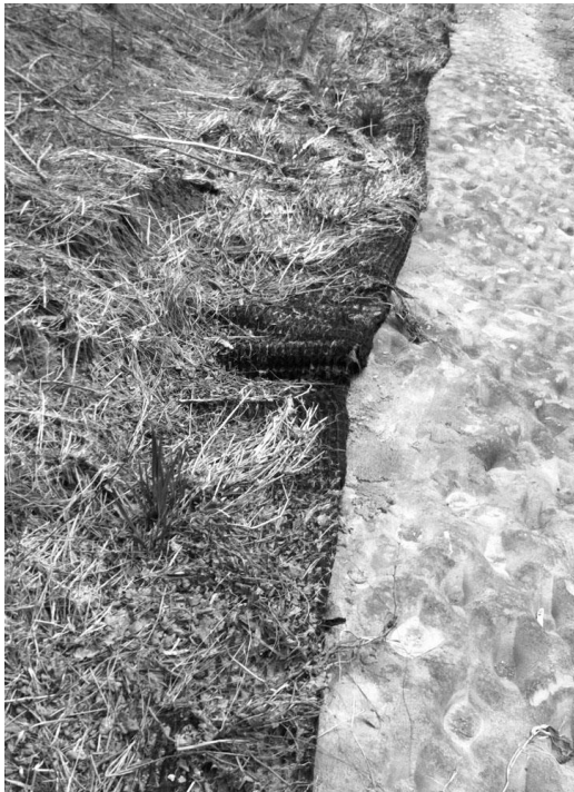
Photo 5. Settled or Eroded Area Along Reach 3
