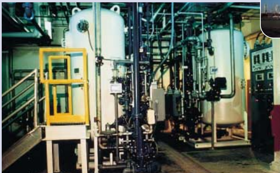
KYNAR® PVDF deionized water (DI) wash system providing superior resin purity.
