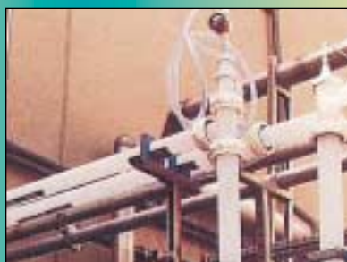
Supply & Return Lines, showing point of ozone injection.
