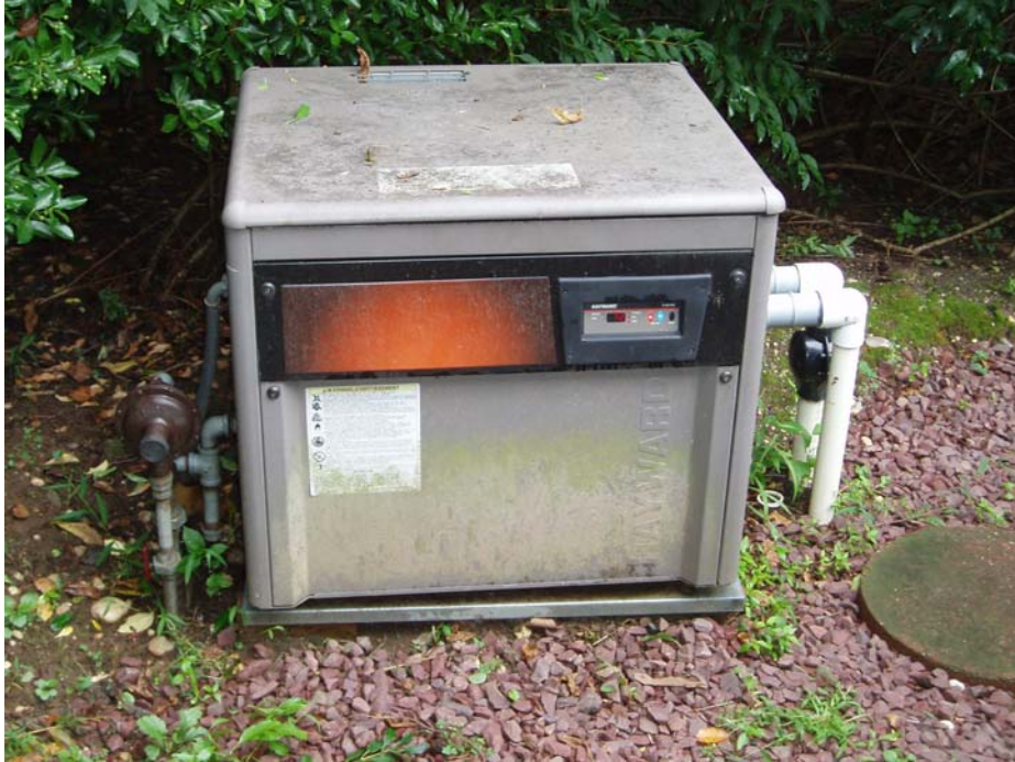
Figure 5 Hayward H-400 induced draft pool heater at the East Northport test site
