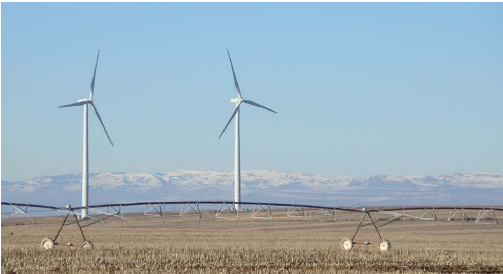
Figure 10: Two of the seven 1.5MW wind turbines at Fossil Gulch Wind Park
