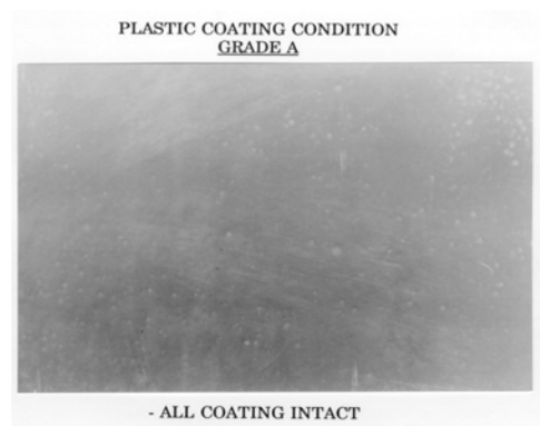
Figure 81 — Plastic coating condition Grade A – all coating intact
