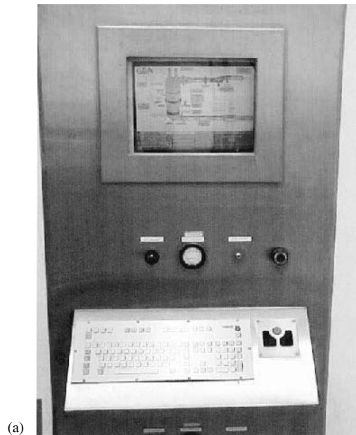
Figure 15 (a) PLC-based control panel. ( continues )
