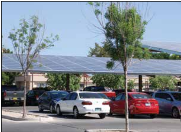
Photo 1.1 • Carport PV systems generate energy and keep cars cool.
