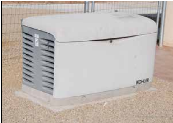
Photo 1.5 • 10 kW backup generator, powered by natural gas, used when utility is out during extended periods of cloudy weather.
