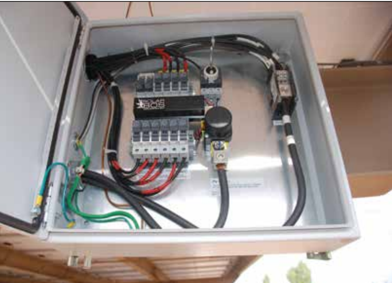
Photo 1.13 • PV combiner with fuses in the positive conductor only. Manual and contactor disconnects in positive conductor only. Not 2017 NEC compliant [690.15(C)].
