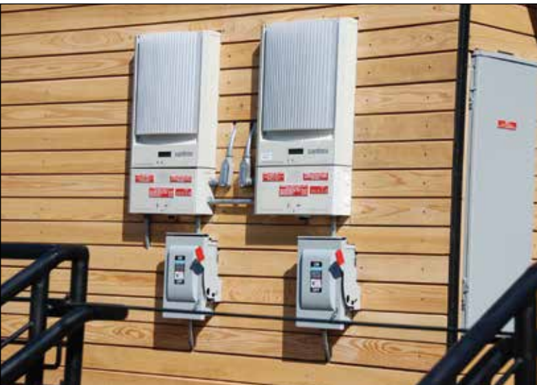
Photo 1.15 • Dual 4 kW utility-interactive inverters.
