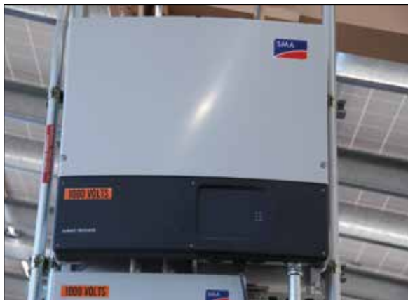
Photo 1.6 • Utility-interactive inverter. External ac and dc disconnects not shown.
