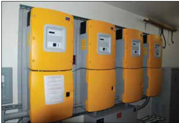
Photo 1.8 • Four 6-kW stand-alone inverters in an ac-coupled, battery-backed-up PV system
