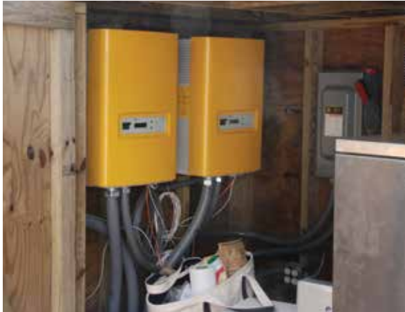
Photo 1.17 • Multimode Inverters. These inverters provide whole-house battery-backed-up energy and are ac coupled to utility-interactive inverters.
