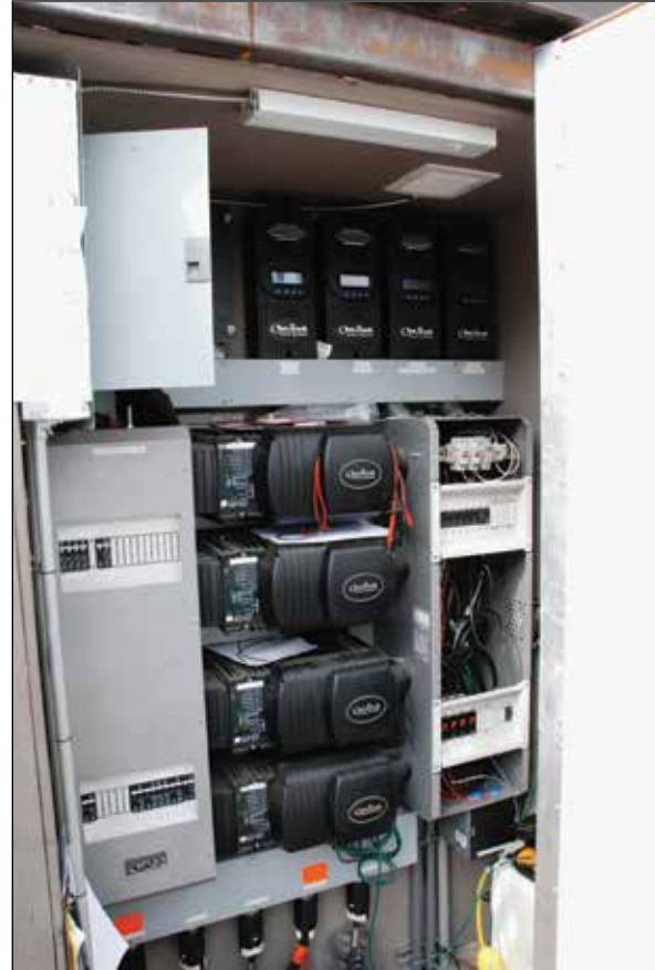
Photo 1.9 • Inverters and charge controllers for 10-kW off-grid, stand-alone PV system.
