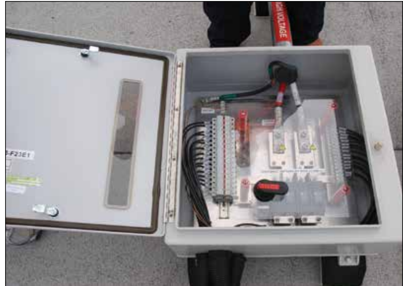
Photo 1.14 • PV combiner in white enclosure with manual switch opening both positive and negative conductors. Plastic shield covers energized, exposed conductors.
