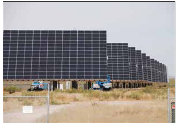
Photo 1.4 • Five mW utility-scale PV system with PV subarrays mounted on two-axis trackers.
