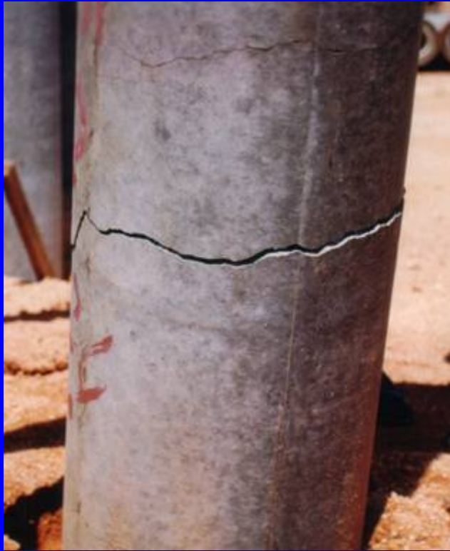
Seriously damaged pile due to severe driving stress in soft ground (tension)
