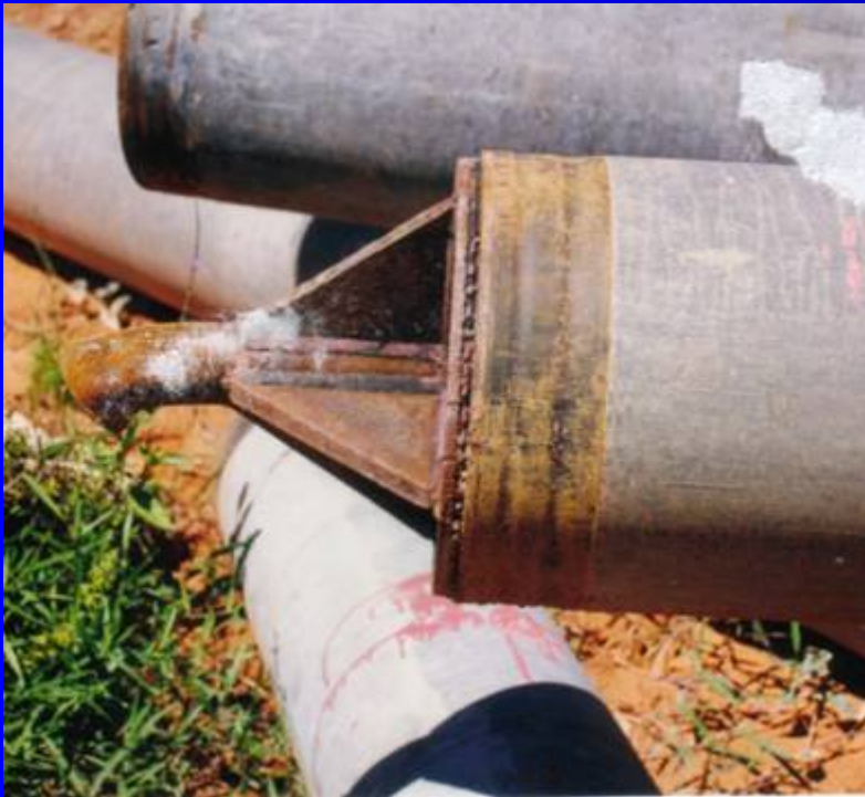
Defective pile shoe
