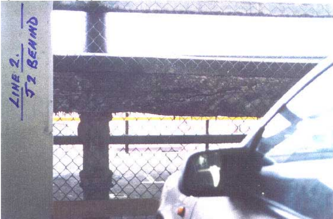
Figure 6.2 - 1 CDM photo [H131] of crack to slab edge at J2, January 1997
