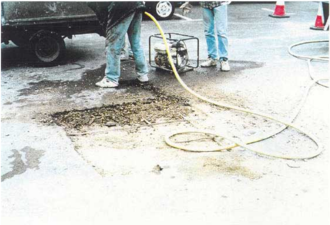
Figure 6.1 - 3 H&S photo [H132] of cutting out for repairs at I2-3, 20 th March 1996.
