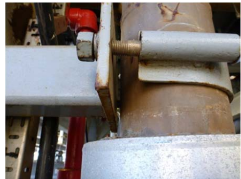
Figure 6 Gap between pipe and support prior to shimming
