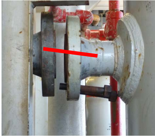
Figure 2: Flange Alignment Problem (discovered after removing bolts)
