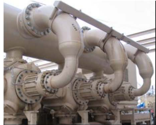
Figure 9 Bracing of cylinder head end unloader piping
