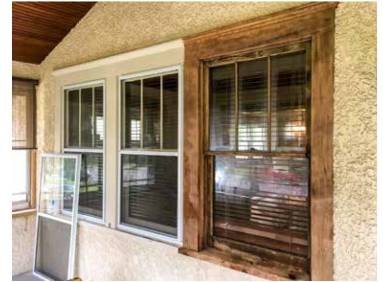
From top: Beginning, middle, and finished project of Jessie's front porch rehab.
