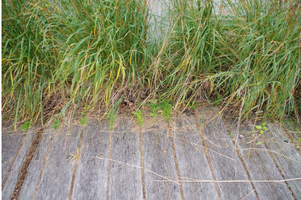
Figure B-3: Plank Rot and Landscape Vegetation on South Trail
