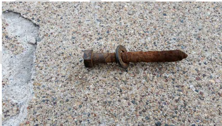
Figure 9: Corroded Bolt that has Lost its Threads
