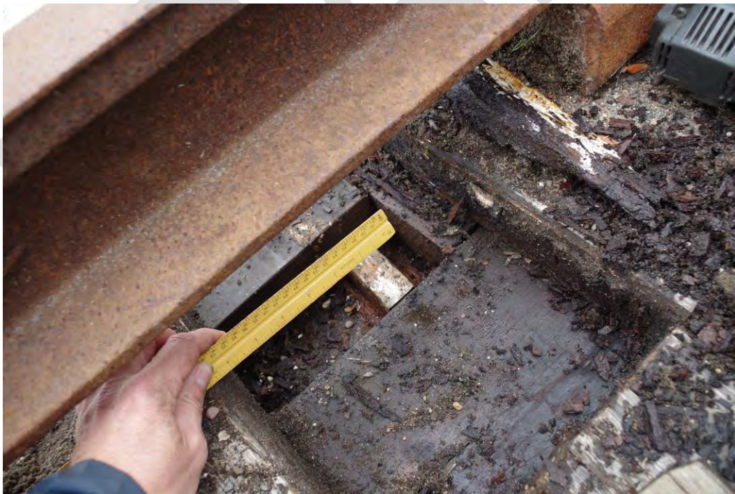
Figure 16: Drainage Hat Channel on South Edge of Trail
