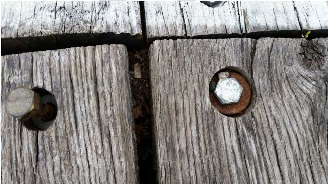
Figure B-6: Loose Countersunk Bolts
