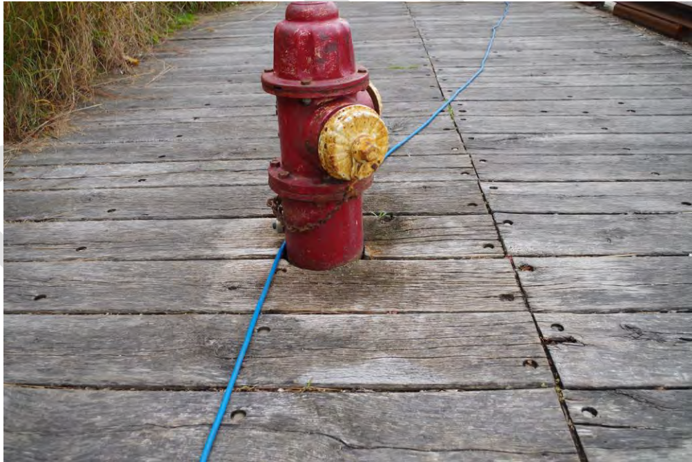
Figure B-4: Wood Rot around Fire Hydrant on South Trail
