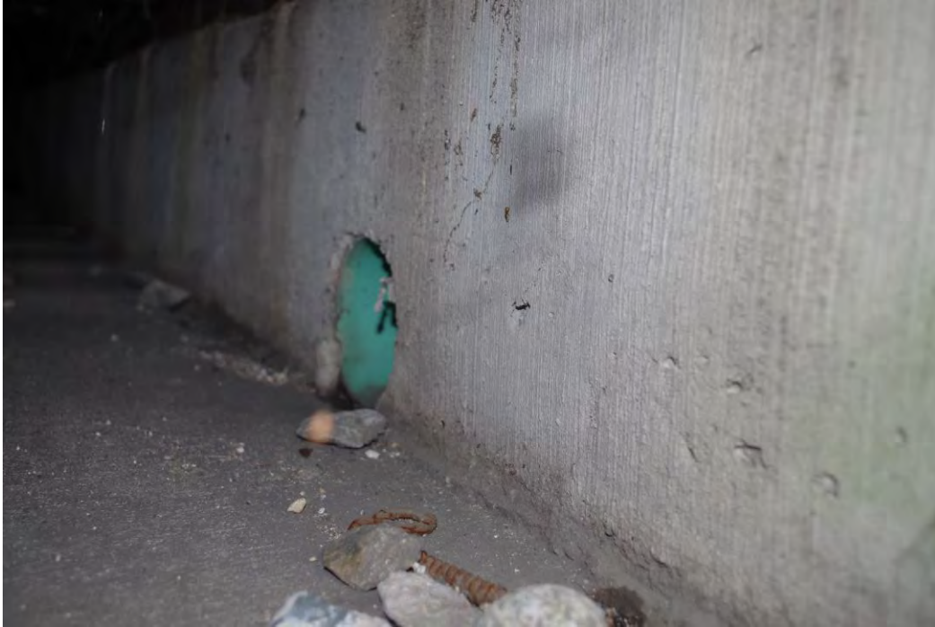
Figure 15: 4-inch Diameter Drain Tile Outlet to Concrete Gutter
