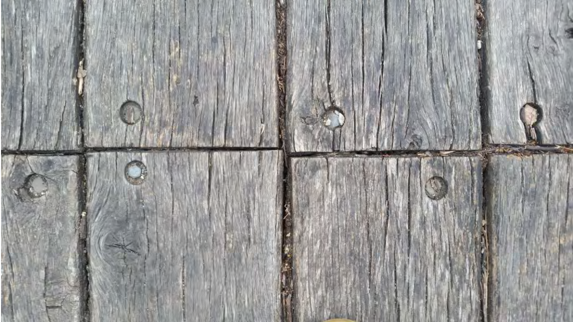
Figure B-8: Countersunk Holes Filled with Debris
