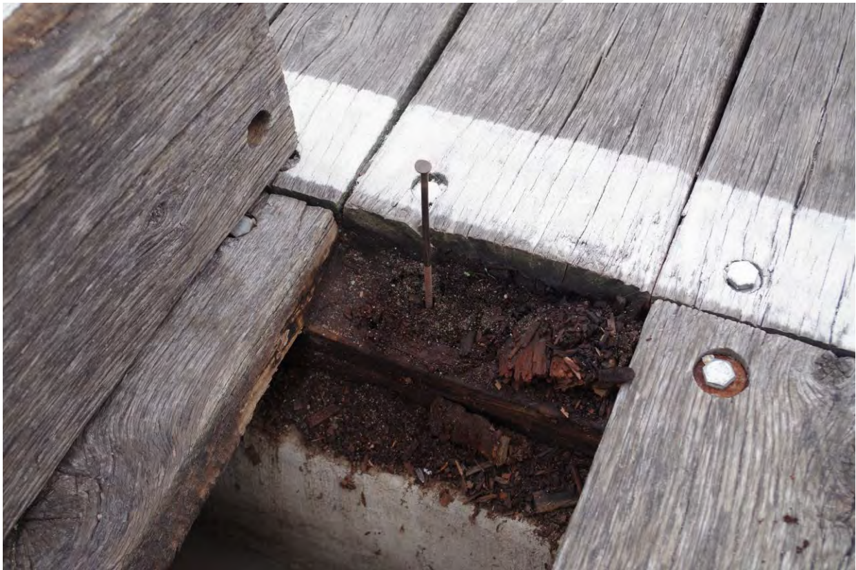
Figure 12: Deteriorated Stringer at North Trail
