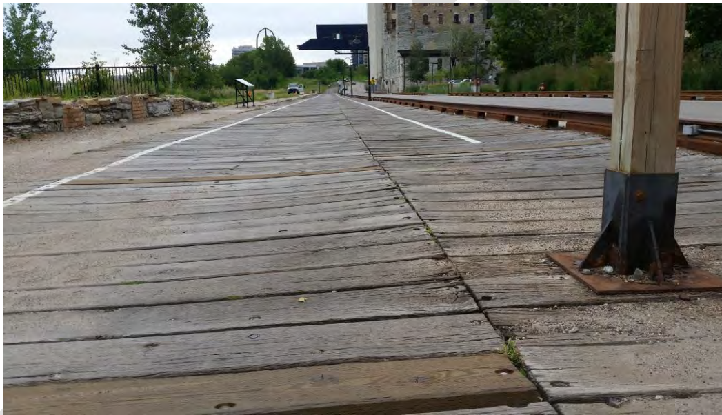
Figure 11: Warping at Butt Seam/Joint in the Center of the North Trail
