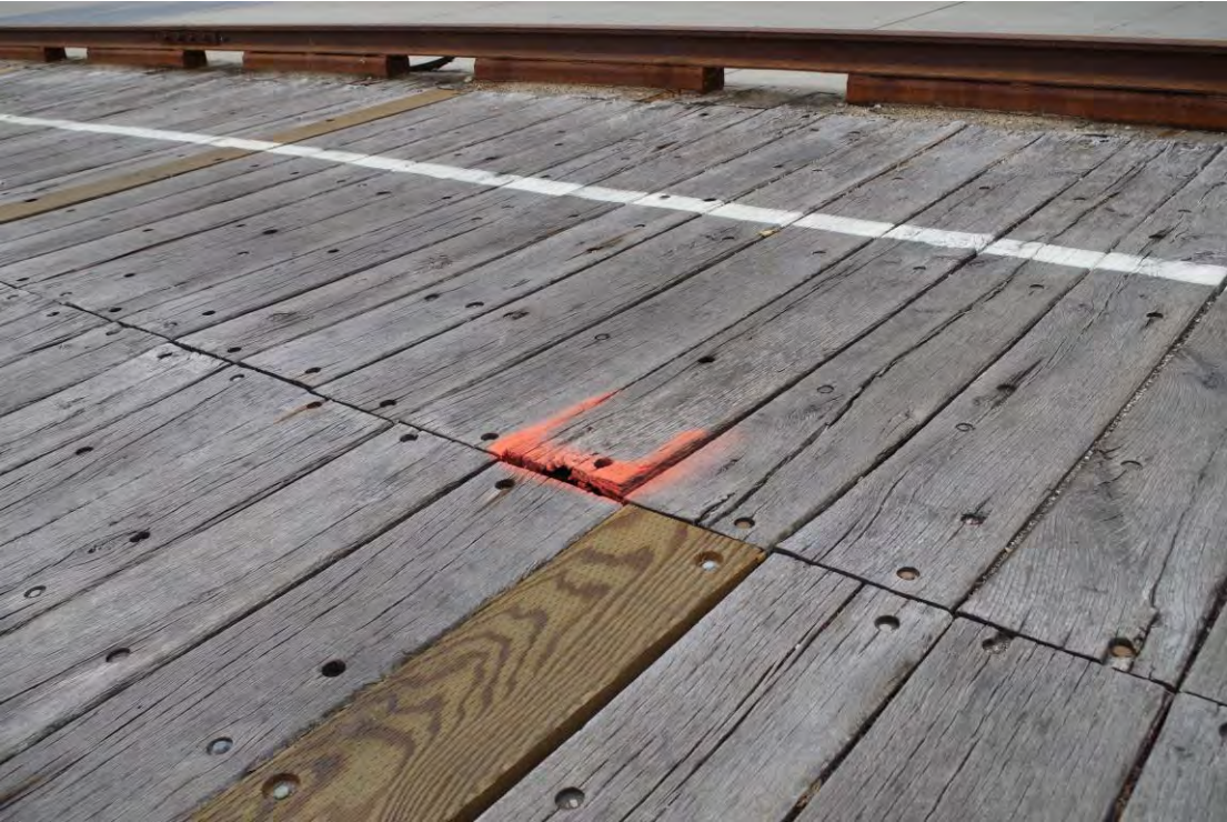
Figure 7: New Plank and Bowed Existing Plank over Butt Seam on North Trail
