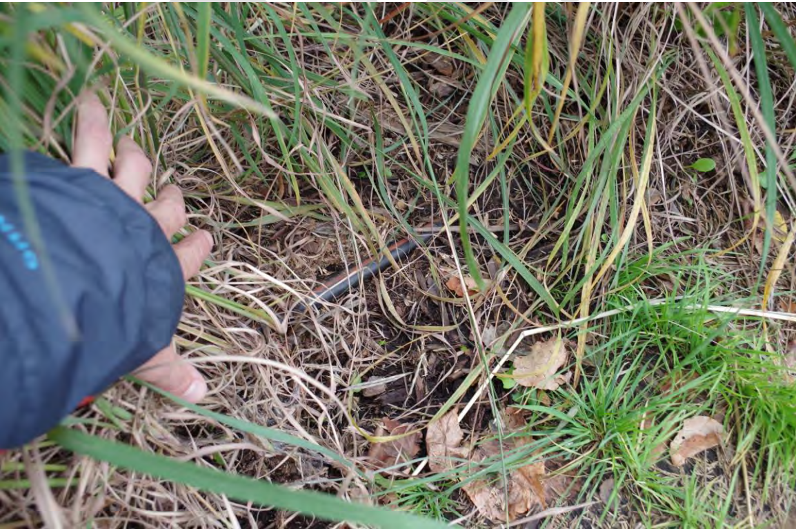
Figure B-11: Sprinkler System on the Border of the South Trail and Adjacent Building
