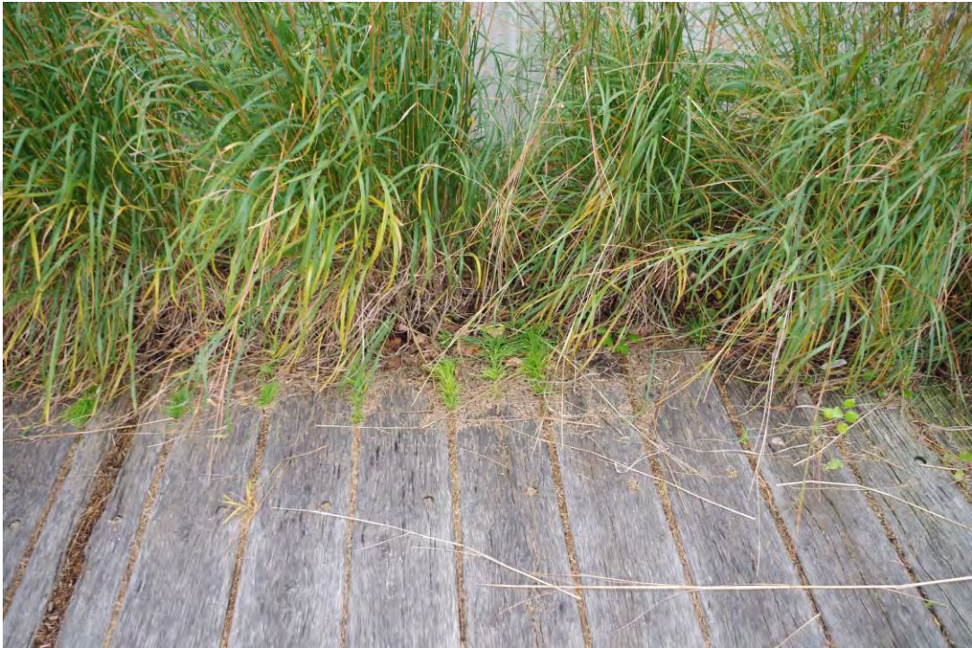
Figure 8: Plank Rot and Landscape Vegetation on South Trail
