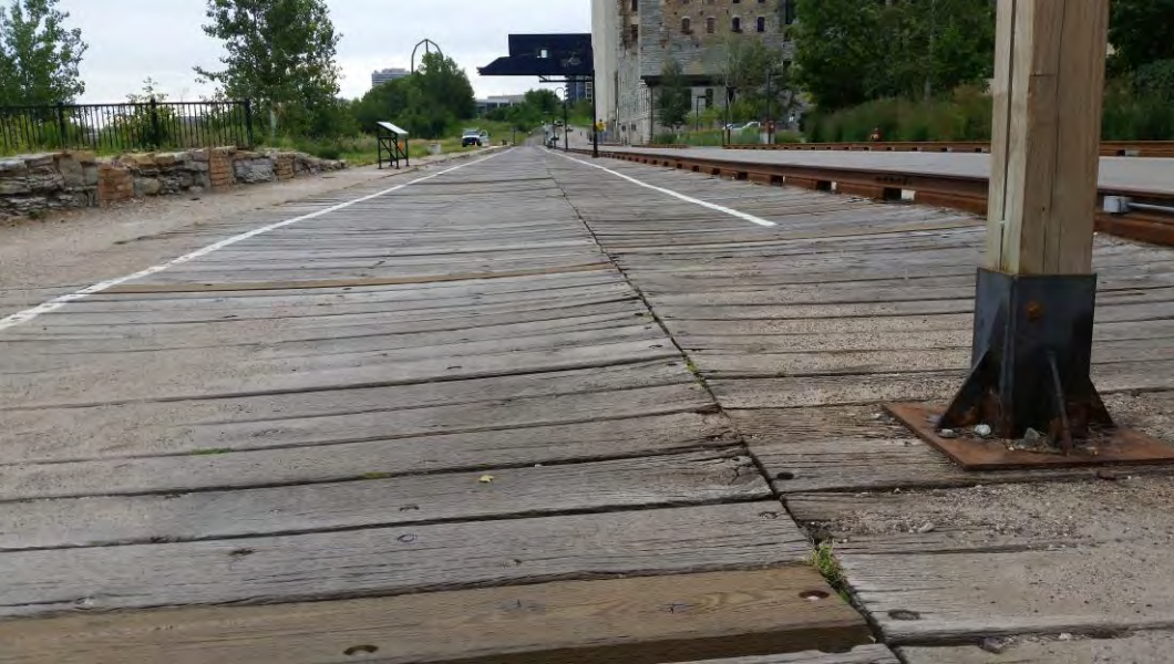
Figure B-7: Warping at Butt Seam/Joint in the Center of the North Trail
