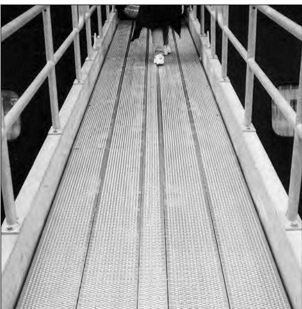
ADA approved TRACTION TREAD™ plank was used to provide a safe, slip-resistant walkway.
