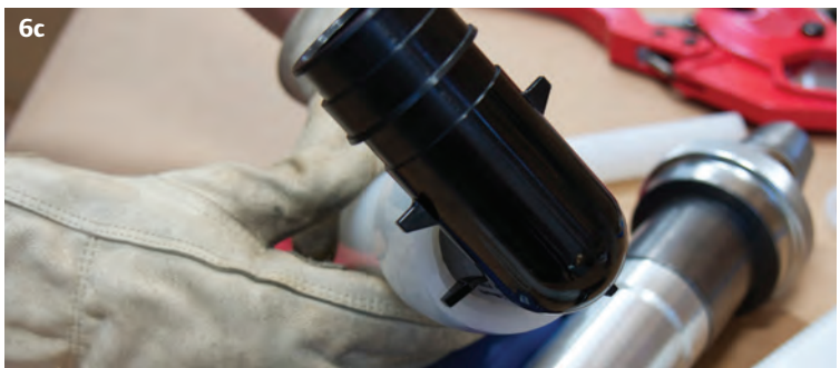
Insert ProPEX Fitting into 2" Uponor PEX Piping.
