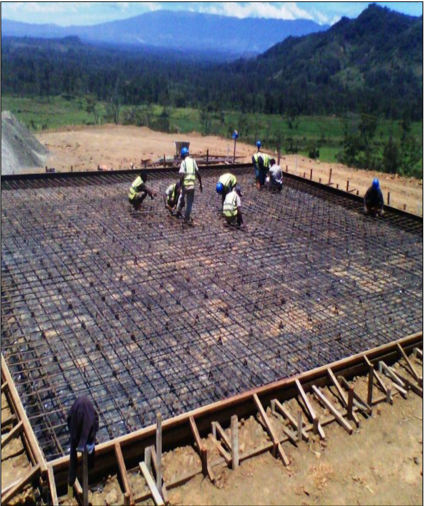
Workers setting foundation for the Southern Cross tank during the construction of new Baisu prison, Mt. Hagen, WHP
