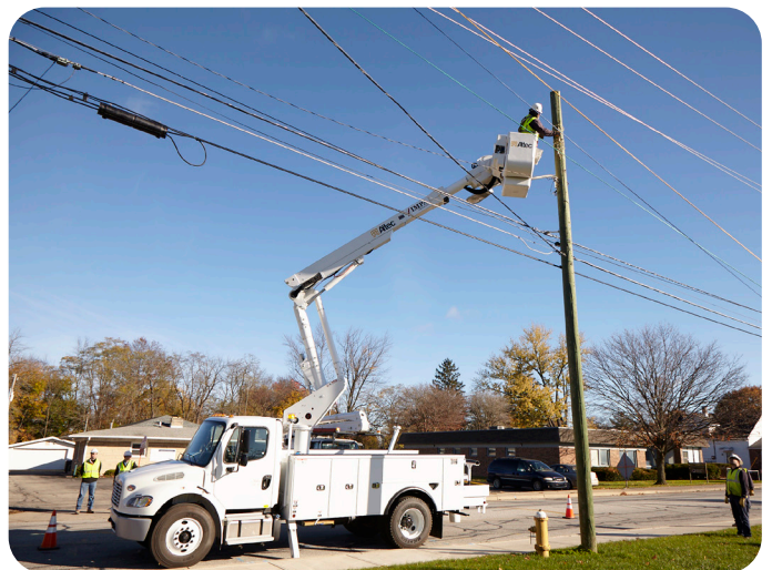
As essential workers, IMPA's crew of lineworkers continued working out in the field to ensure essential access to power.
