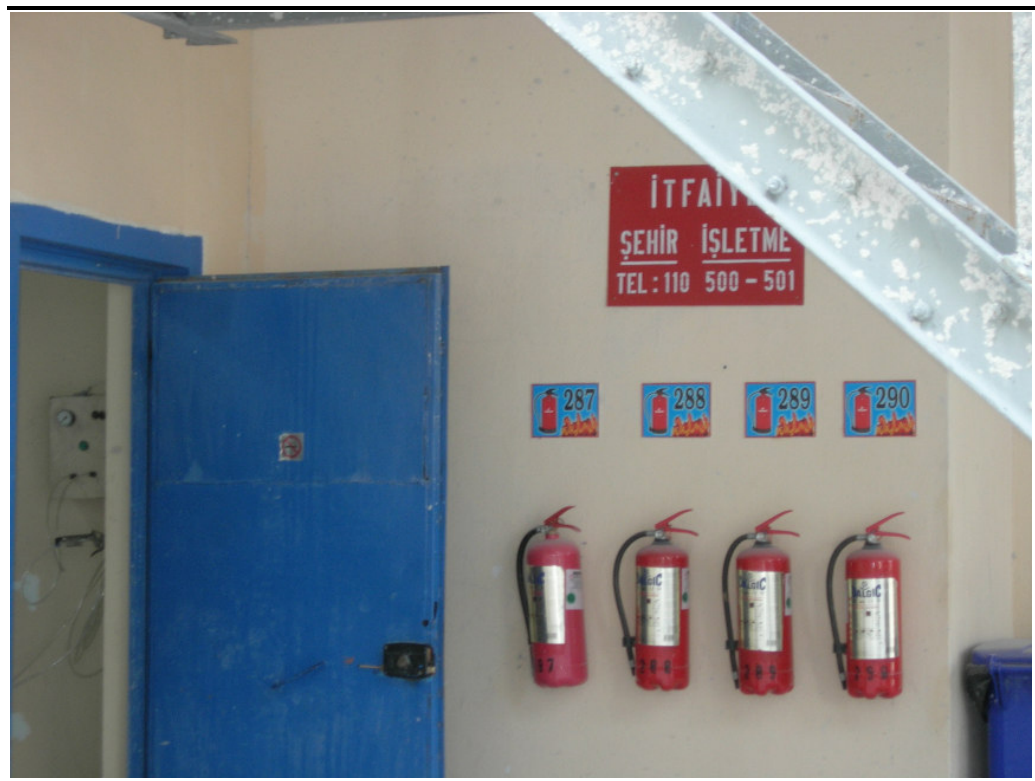
Box 1.16 ETI Health and Safety Management
