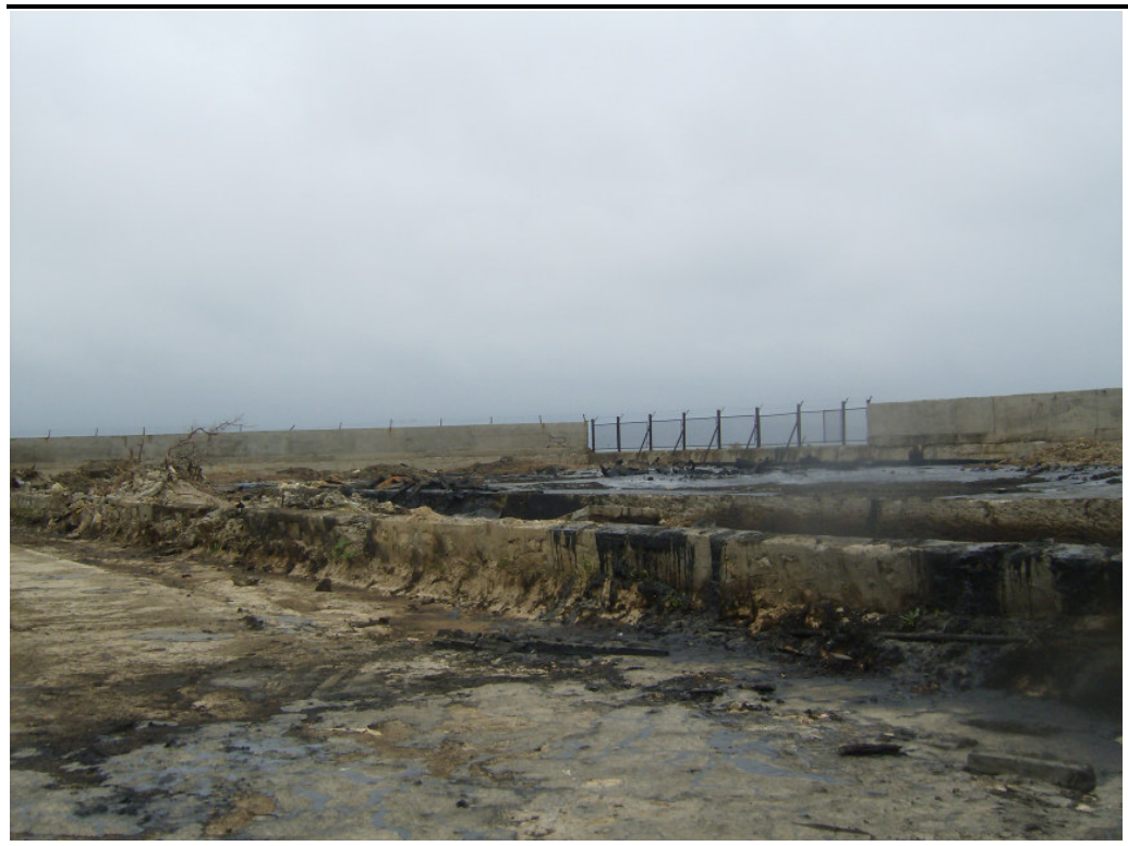
Box 1.11 Contamination from the Removal of Acid Tanks
