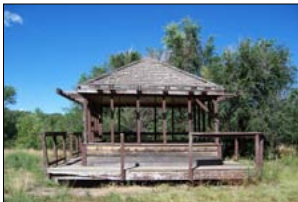
Fire tower platform to refurbish for trail-spur destination lookout point at Running Deer
